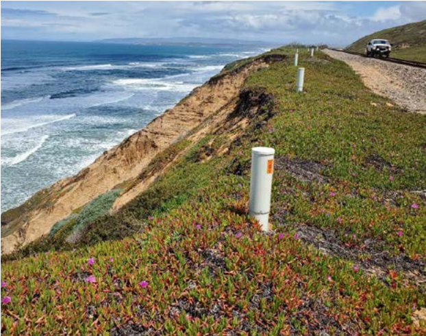
Visible coastal erosion adjacent to the tracks at the Honda Bluffs in Santa Barbara County.
